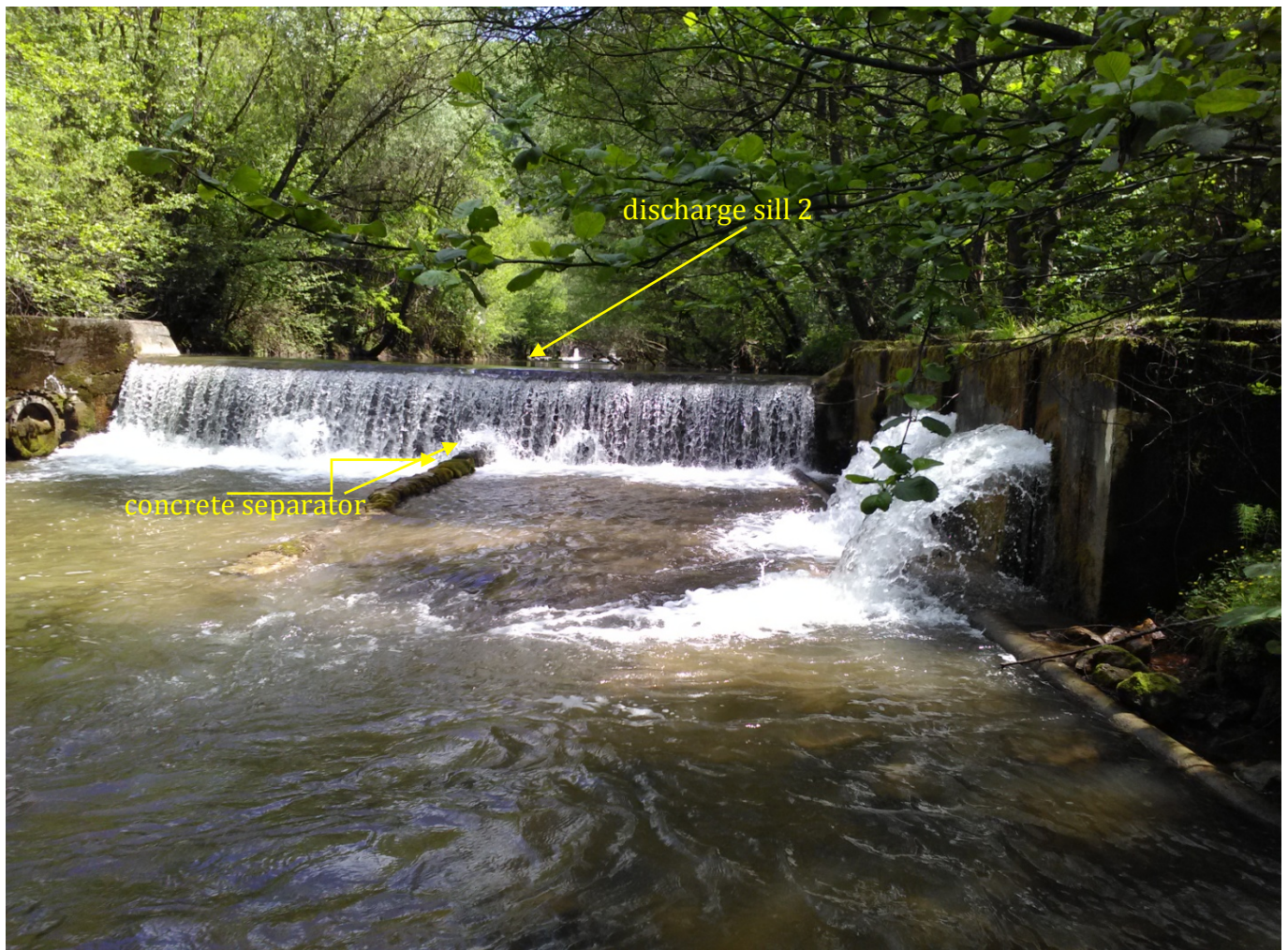
Figure 3. The discharge weir at site 2, showing the existing concrete separator - indicative figure.
